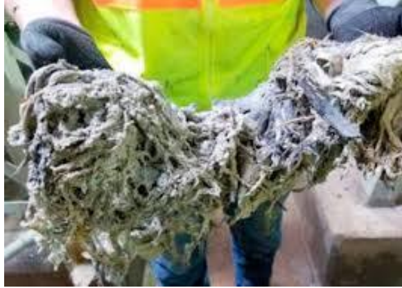
Photo: a sewer worker holding a large mass of "flushable" wipes that were clogging a sewer pipe
