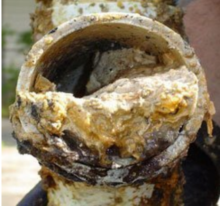
Photo: a sewer pipe half full of congealed grease
