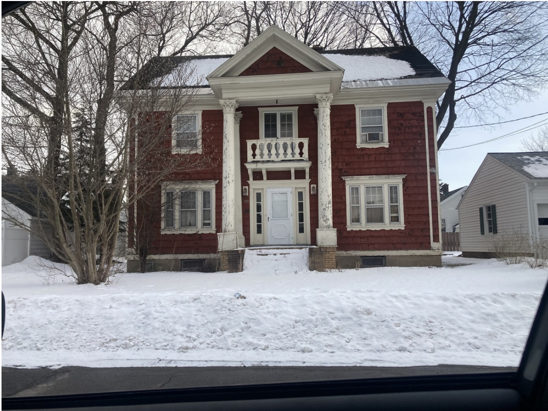
A property at 2803 that has been vacant for several years, much to the dismay of the neighbors.
